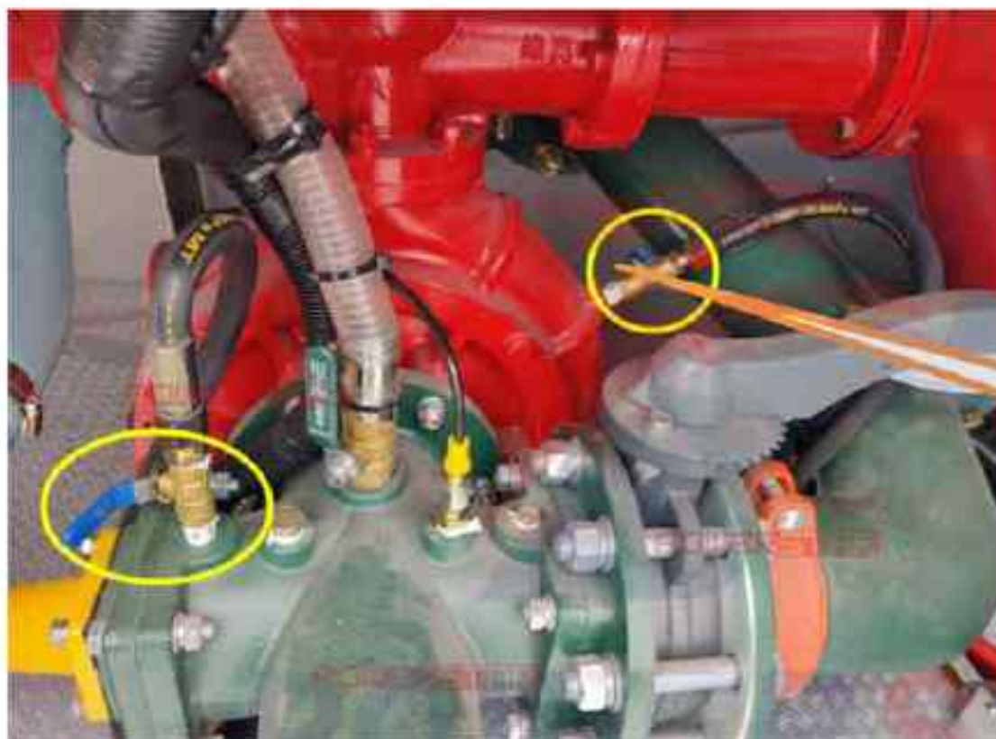
Inlet and Outlet valve for cooling system
