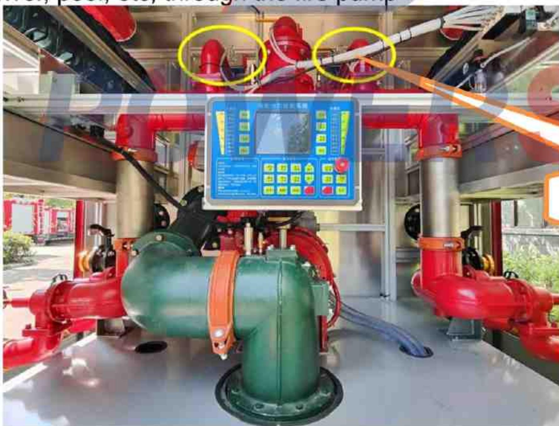
Water Inlet Control Valve:
